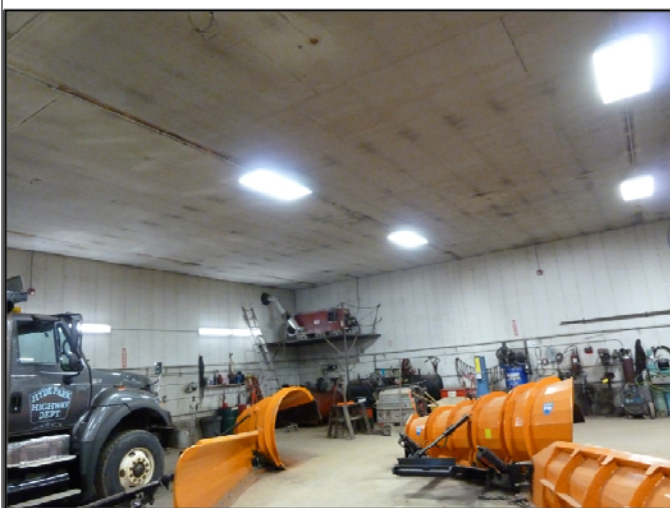
Energy efficient lighting installed in the Hyde Park Town Garage
