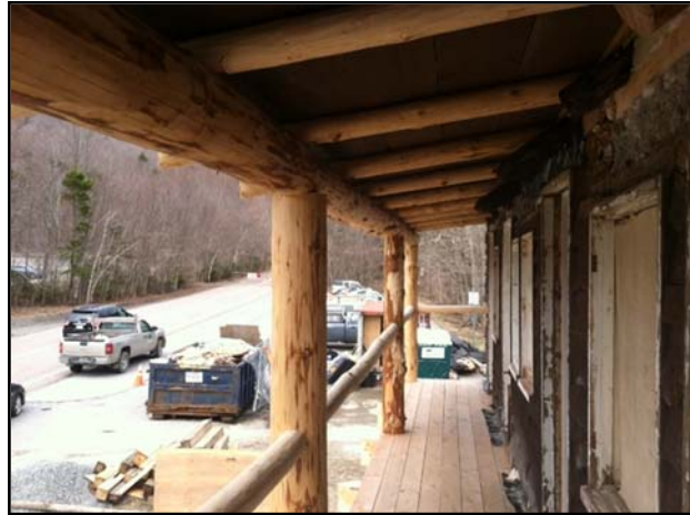
Restoration of the second floor porch is almost complete. The porch was restored using Vermont grown spruce beams and will look much like it did when the Camp was first built in 1927.
