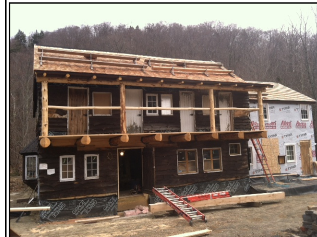
Barnes Camp is looking like its old self! The “south wing,” reconstructed based on historic photos, is awaiting siding. The “south wing” will house much needed restroom facilities and a water collection system.
