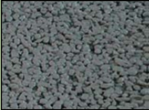
Porous concrete surface
