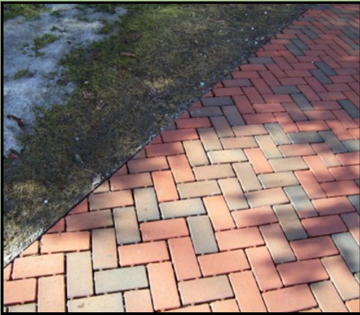
Permeable pavers installed at the State of Vermont Forensics Lab in Waterbury
