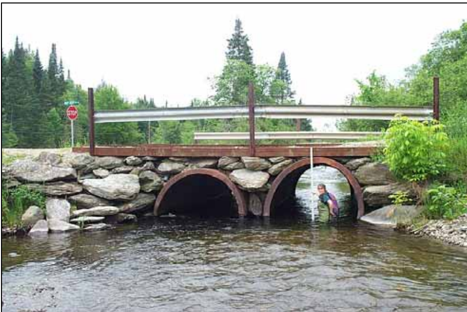
Twin culverts in M18-A high priority for replacement
