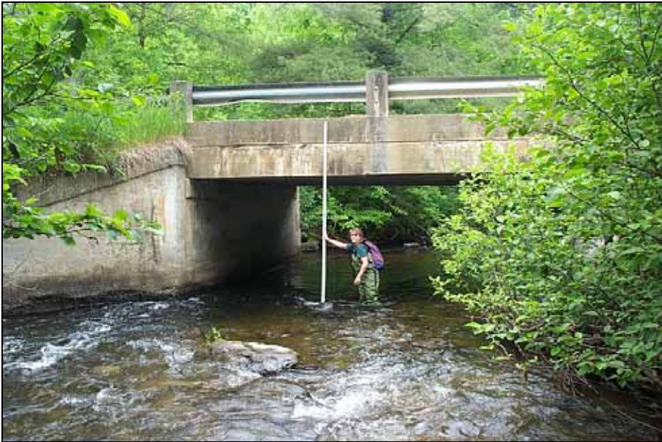
Undersized bridge in M18-B identified as a priority for replacement
